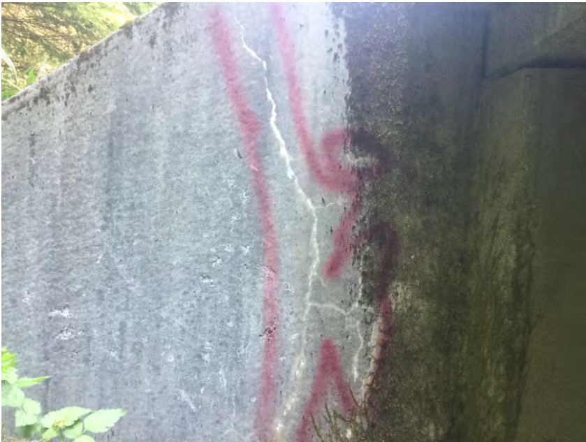
Hairline cracks noted on right ballast wall
